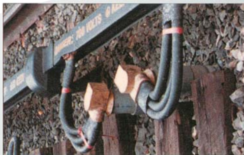
Third Rail Insulation and Termination Connectors
