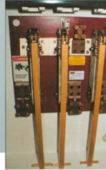
Three Knife Blade Switches in Cabinet
