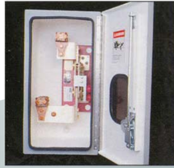
1200 Amp Voltage Pressure Switch in Fiberglass Enclosure
